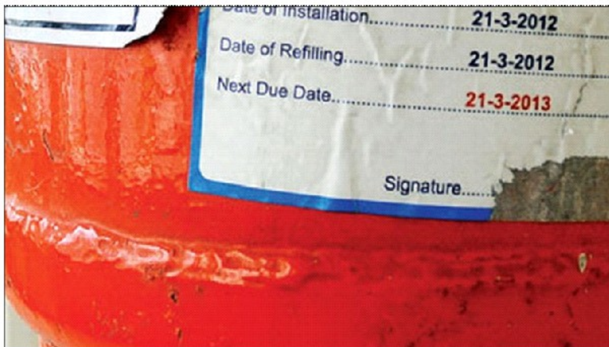
Fig 3.4.1.3 Know the refill date on the fire extinguisher
